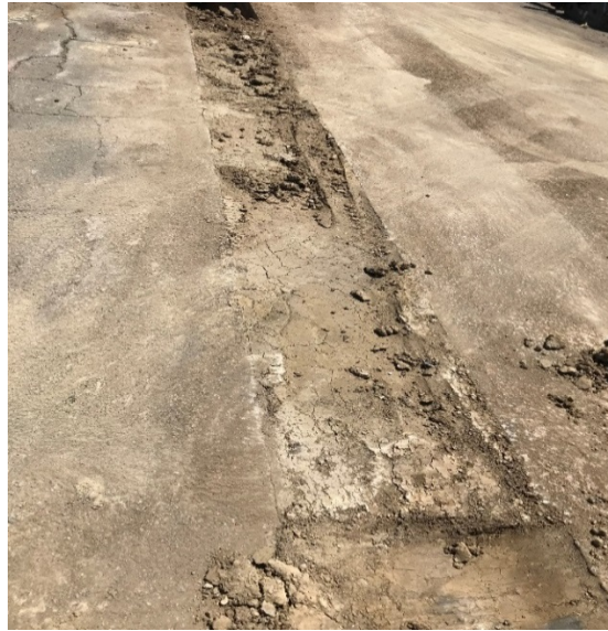
Figure 10. Denver Street Test Site in Pueblo, CO.
